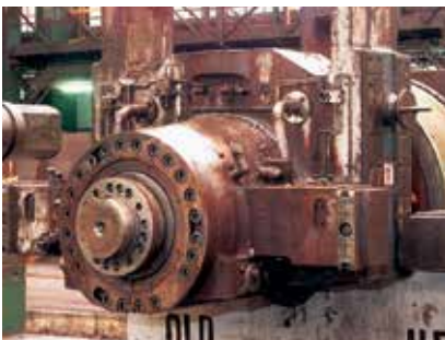
Thrust collars on bearing chocks create higher preloads than the previous method and therefore even the heaviest peakloads can be absorbed. The roll necks are lasting and the production runs smoothly.
