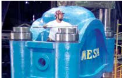
Eight Superbolt column nuts required only 12 man hours for installation vs. 2-1/2 full days for heating of columns.
