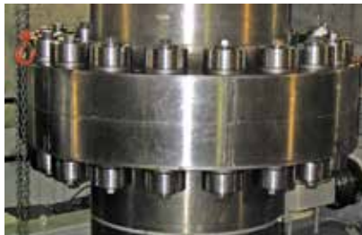
Superbolt expansion bolts are ideally suited for shaft couplings, as seen here on this Francis type pump/generator shaft coupling at a pumped-storage facility.
