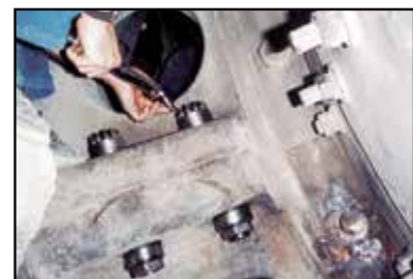
Split gear segment on rotary kiln.
